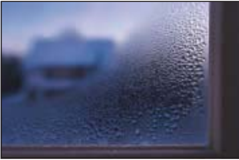
Condensation on the inside of a windowpane.
